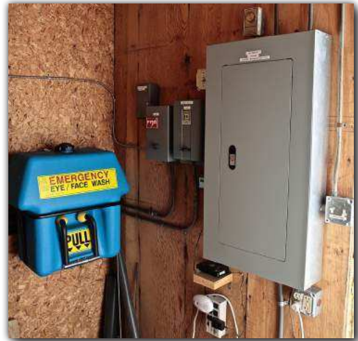
AE - 12 Control Panel
