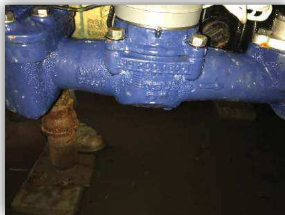
AE- 47 Flow Meter
