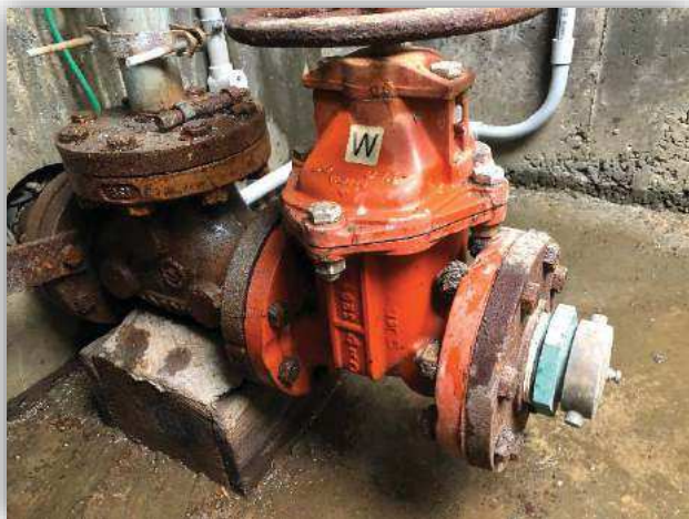
AE- 68 Blow off valve
