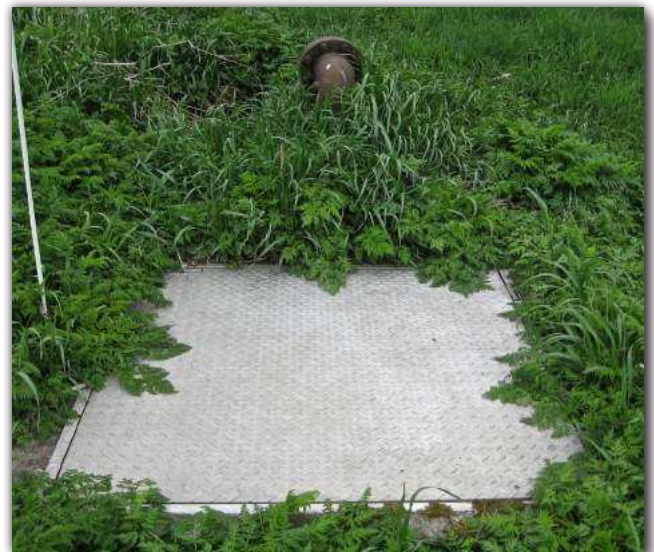
AE - 20 Valve Vault Access Hatch
