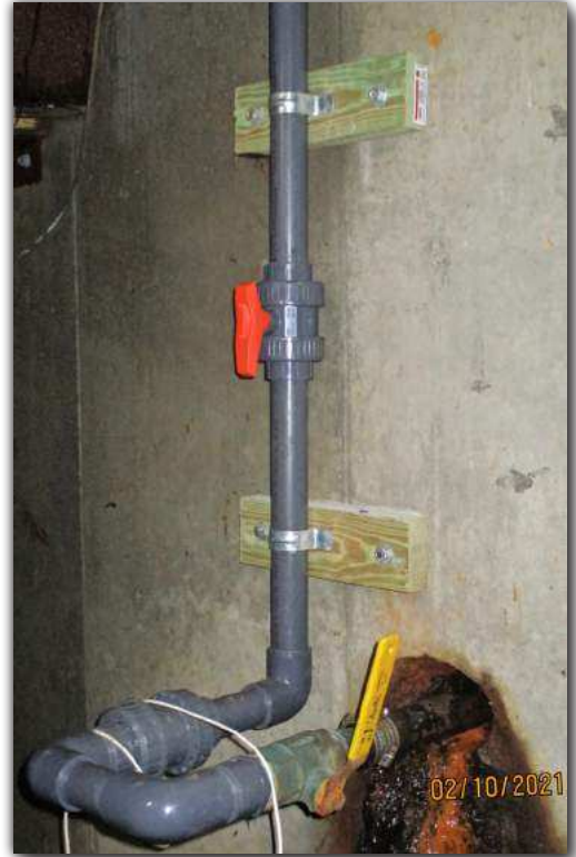
AE - 16 Discharge Piping
