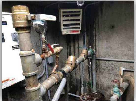
AE- 73 Heater and piping
