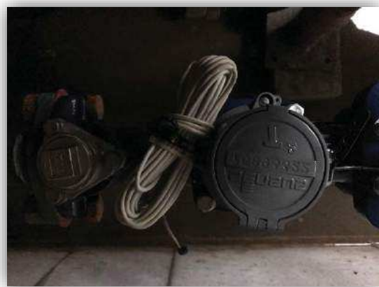
AE- 45 Flow Meter
