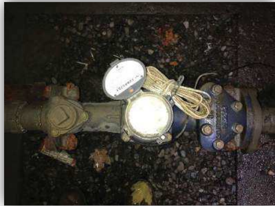
AE- 59 Flow Meter
