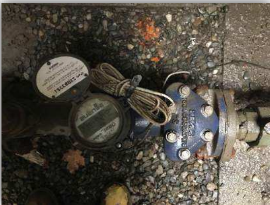
AE- 60 Flow Meter
