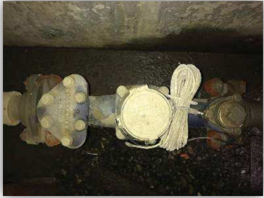
AE- 57 Flow Meter
