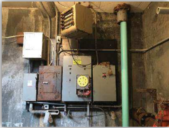
AE- 96 Control Panel
