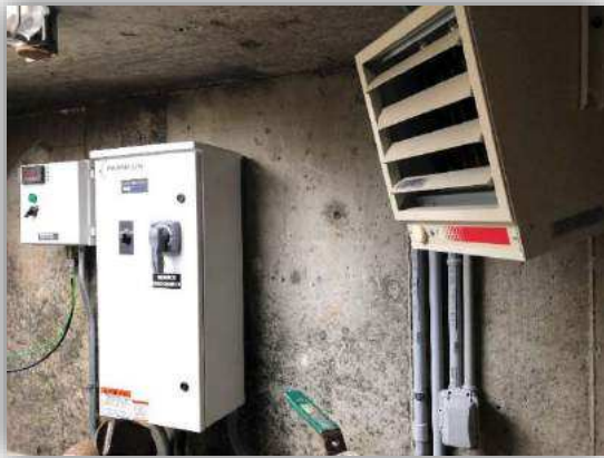
AE- 72 Heater and panel
