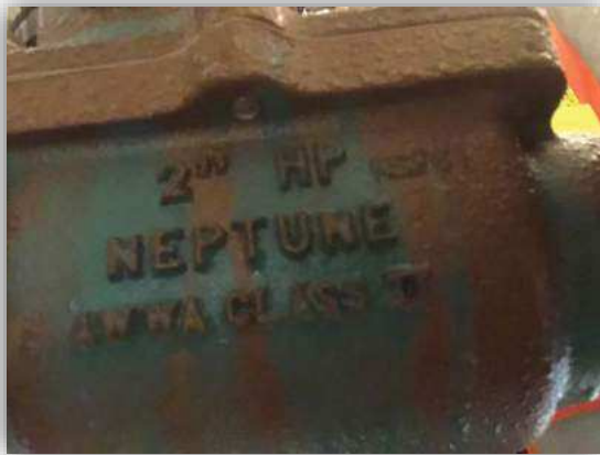
AE- 86 Flow Meter
