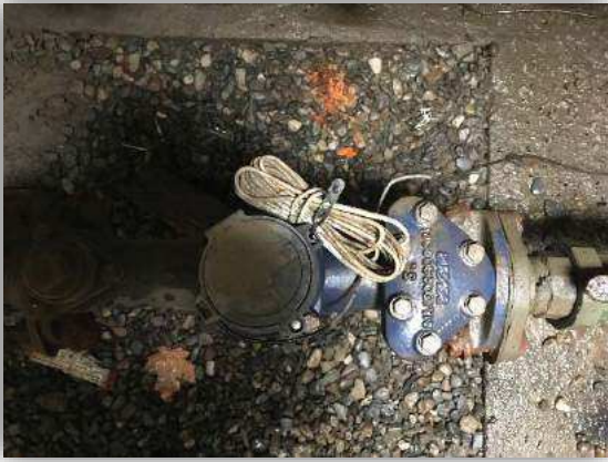
AE- 56 Flow Meter
