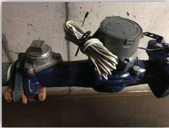
AE- 44 Flow Meter
