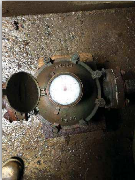
AE- 110 Flow Meter
