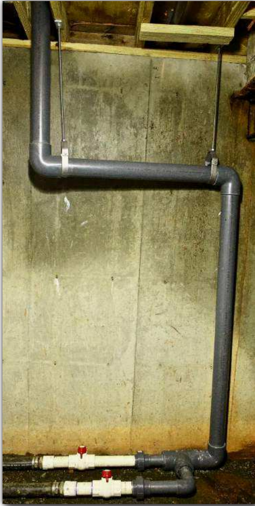
AE - 15 Inlet Piping
