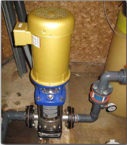
AE - 5 Fire District Pump No. 1
