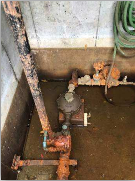
AE- 114 Well Piping
