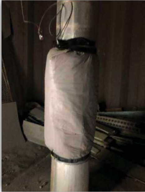
AE- 126 Insulated Piping
