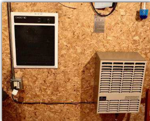
AE - 17 Heating Units
