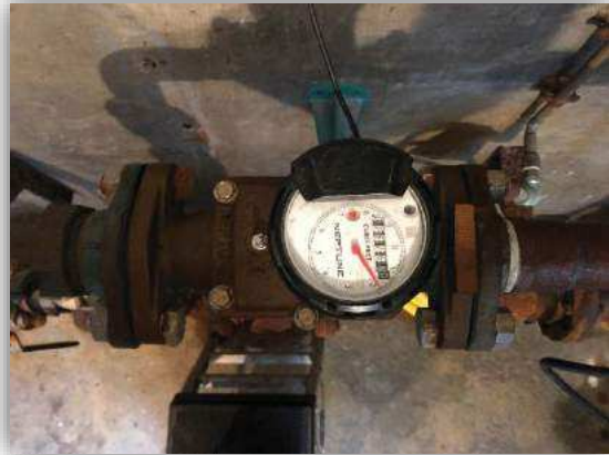
AE- 85 Flow Meter
