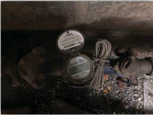
AE- 58 Flow Meter
