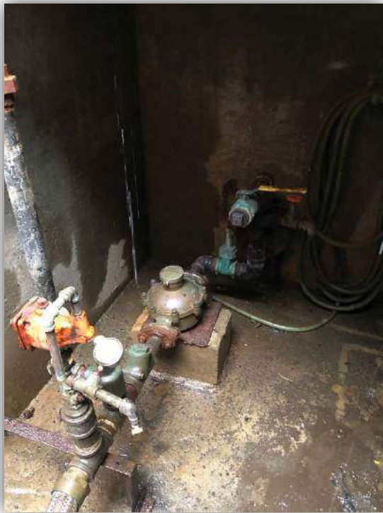
AE- 112 Well Piping
