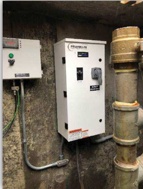
AE- 65 Control Panel
