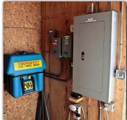
AE - 10 Control Panel
