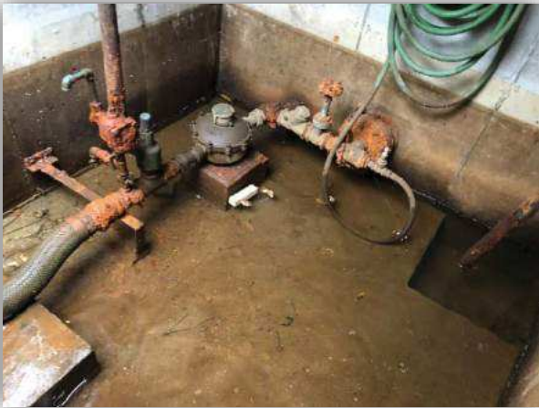
AE- 116 Well Piping
