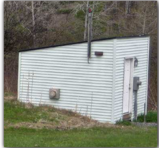
AE - 1a Fire District Pump House
