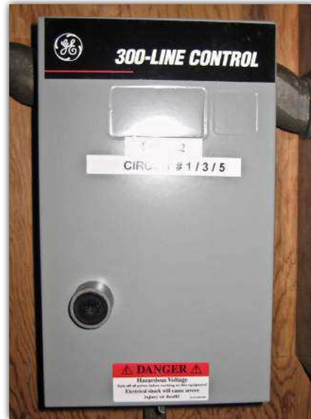
AE - 14 Pump Control
