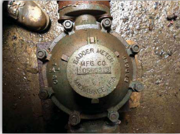
AE- 111 Flow Meter
