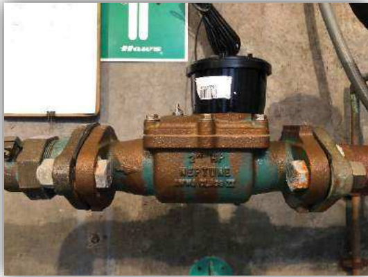
AE- 84 Flow Meter
