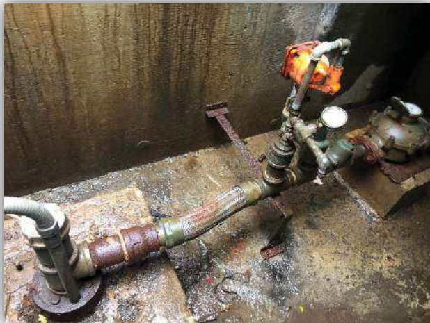
AE- 108 Well Piping
