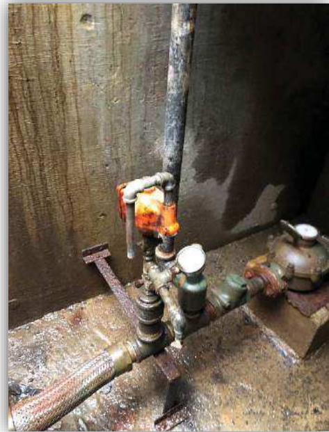
AE- 109 Well Piping
