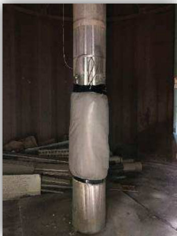
AE- 124 Insulated piping
