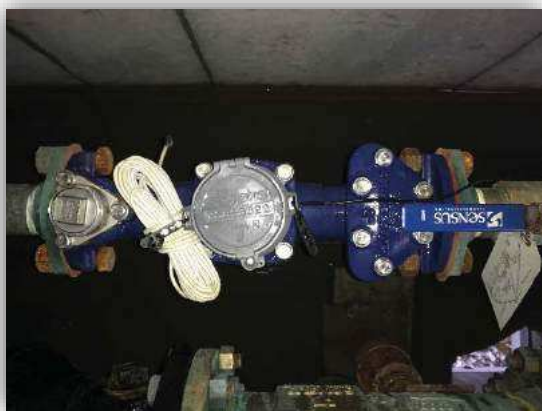
AE- 46 Flow Meter
