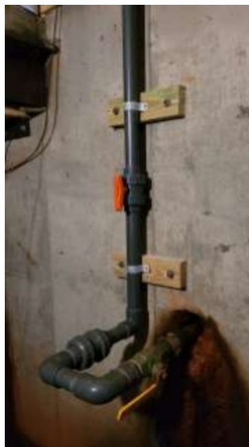
Shut-off valves in basement of Treatment Building
