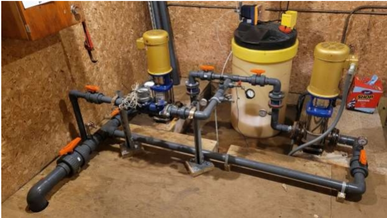
Chlorination Day Tank, Pumps, Piping Flow inside Treatment Building
