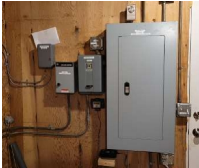
Timer, pump switch and circuit breaker panel box in Treatment Building
